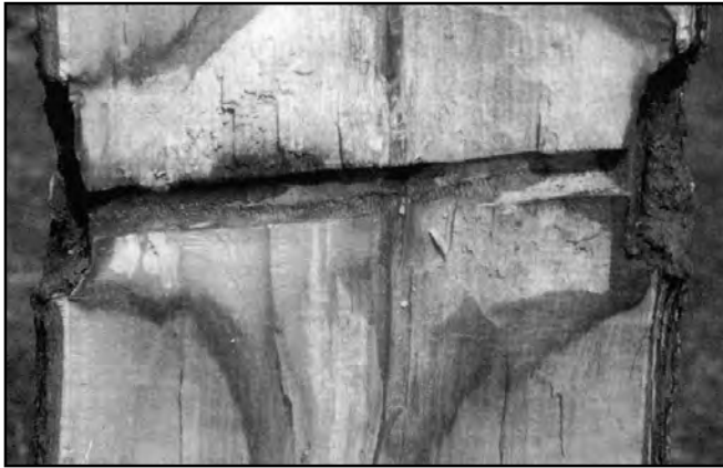
Figure 3. Longitudinal view of discoloration and decay extending from drill hole for hardware installation (note countersinking of washers into wood) (Stobbe et al. 2000).
