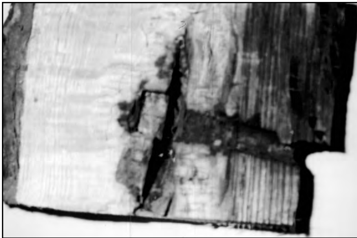
Figure 7. Red oak showing discoloration associated with drilling a hole for through-hardware installation (37 years since installation). Wall four prevented discoloration from extending into callus tissue, even though the nut and washer were not completely callused over for 8 years after the initial installation (compare Figure 8).
