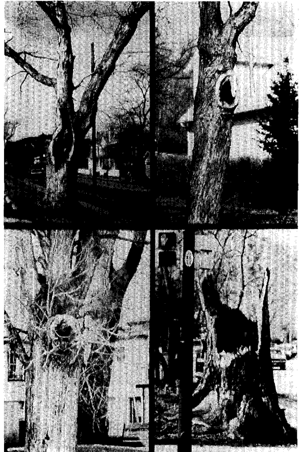
Figure 1. To improve tree health and reduce potential liability, dead parts of trees are removed. In the process structural defects may be revealed, sometimes too late.
