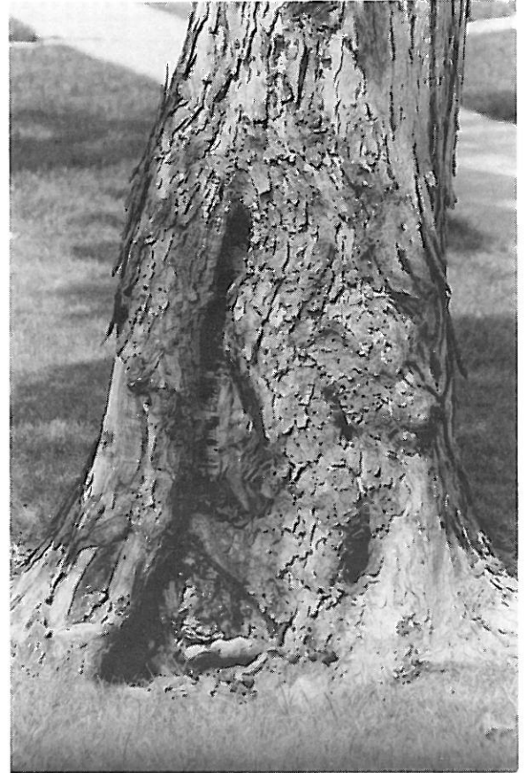
Fig. 5. Trunk damage caused by careless construction workers while installing a water main in the parkway.
