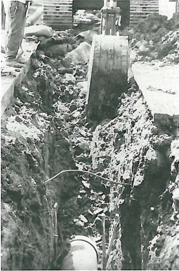
Fig. 2. Construction damage to the root system of a parkway tree during installation of a sewer.
