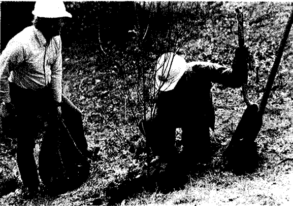
Figure 1. Replacement of a removed tree with a dogwood in the utility right of way.
